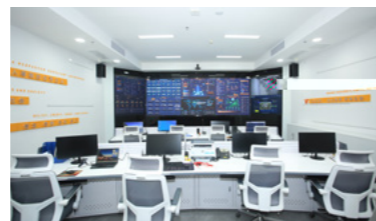
Computer room and monitoring room of main data center of the Group
